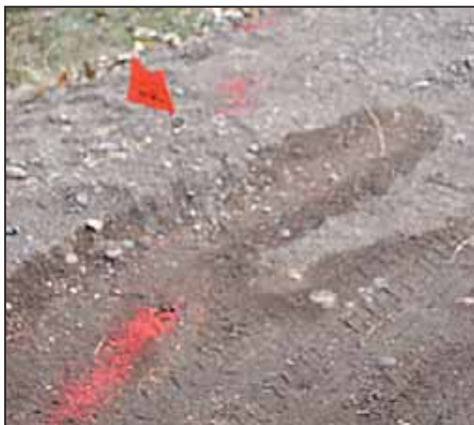
Locators use flags, paint or other colored markers to clearly show where a buried utility line runs. Different utilities use different colored markers to show a location.
