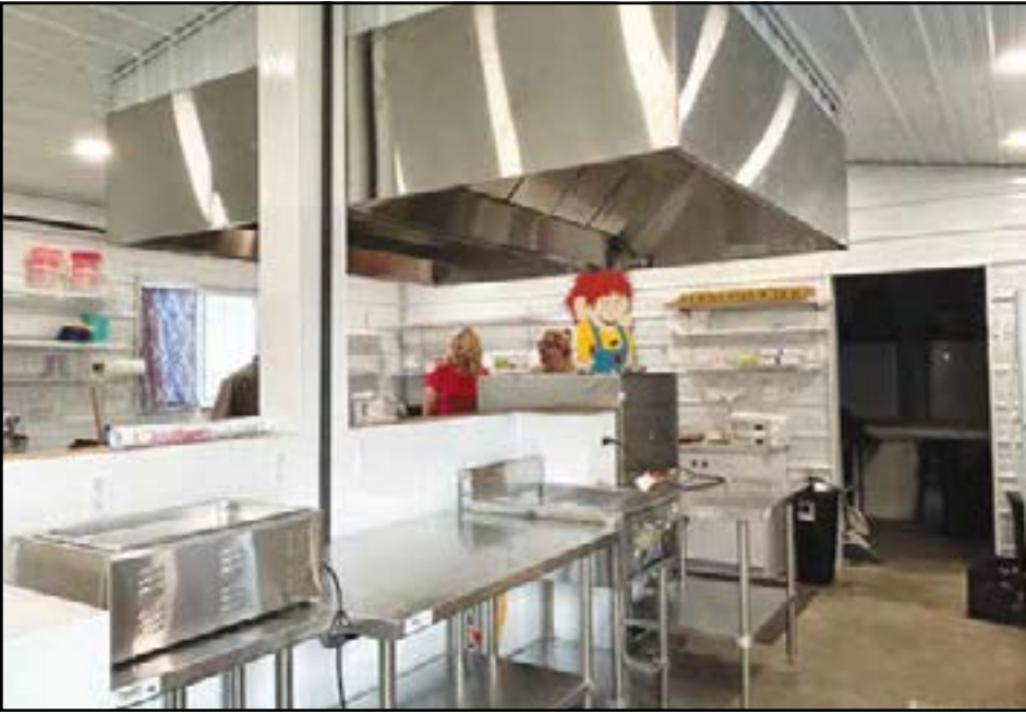
All new equipment for the Sons of Norway fair booth has been installed and ready to fry up the Vikings and Norskies for the 2023 fair. Commercial fans and new grease fryers will curtail the heat emissions in the booth.
