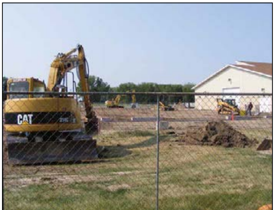
The addition to the Richland County Event Center will still be under construction during the 2023 Richland County Fair but fair staff are doing everything in their power to not allow it to interfere with the fair goer's experience. (Photo by Jaymi Mozeak)
