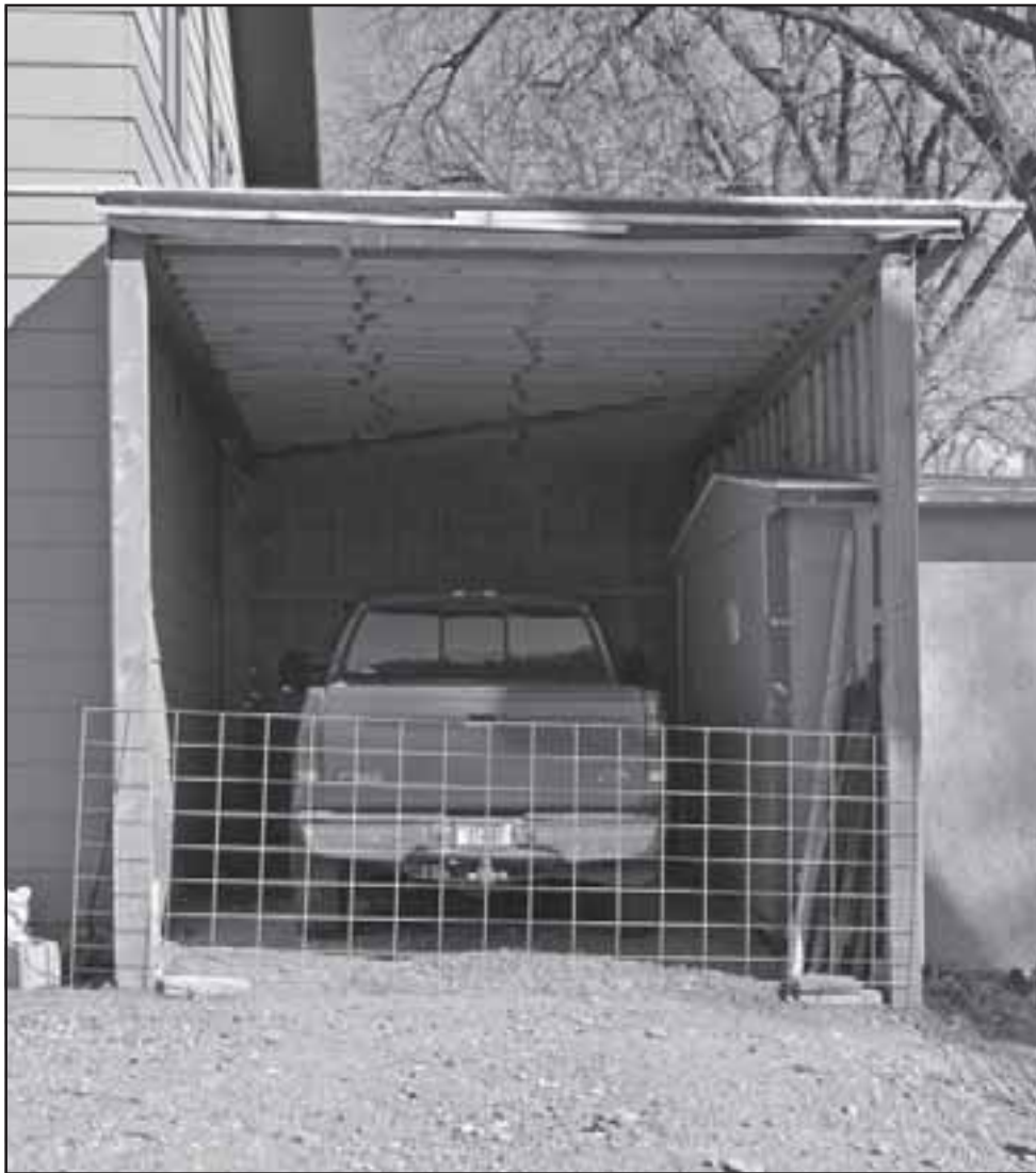
Below: The completed carport. Now we roll up our sleeves for the second portion of this project.
