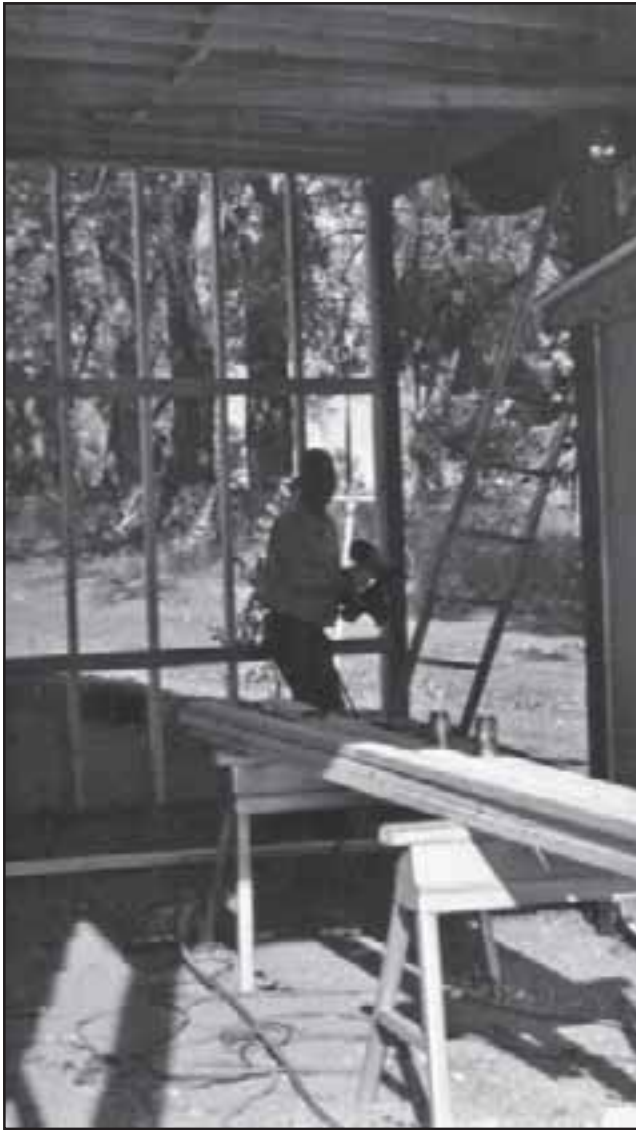
Right: After completing the roof, we closed in the north and east ends of the carport.
