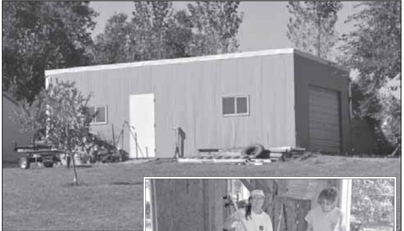
Above: The shop looks practically the same on the outside as it did before we started work, but oh my, what a difference a new roof and a replaced wall can make on the inside of a building.
