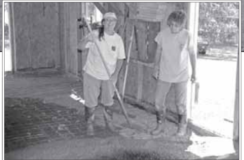
Friends and relatives helped to pour the cement floor, the first order of business in restoring the old building.
