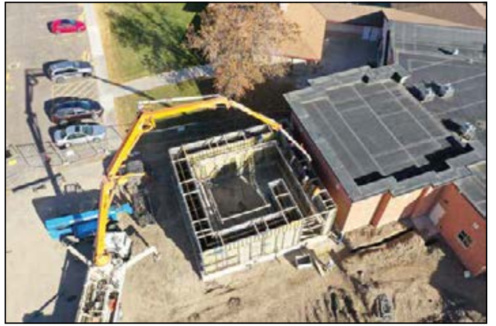
The second radiation vault will be ready in October 2023, the new TomoTherapy machine will be installed in December 2023, and the unit will be ready for patients in January 2024. (Photo submitted by Sidney Health Center)
