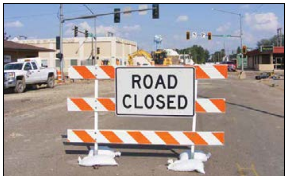
The construction crews that started tearing up Lincoln Avenue in April to work on the water mains have moved on to Central Avenue just a few weeks before July 4. (Photo by Jaymi Mozeak)
